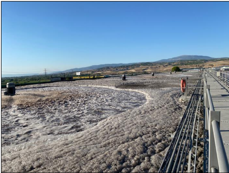
Figure 4.21 Photographs of Existing WWTP in DOIZ
